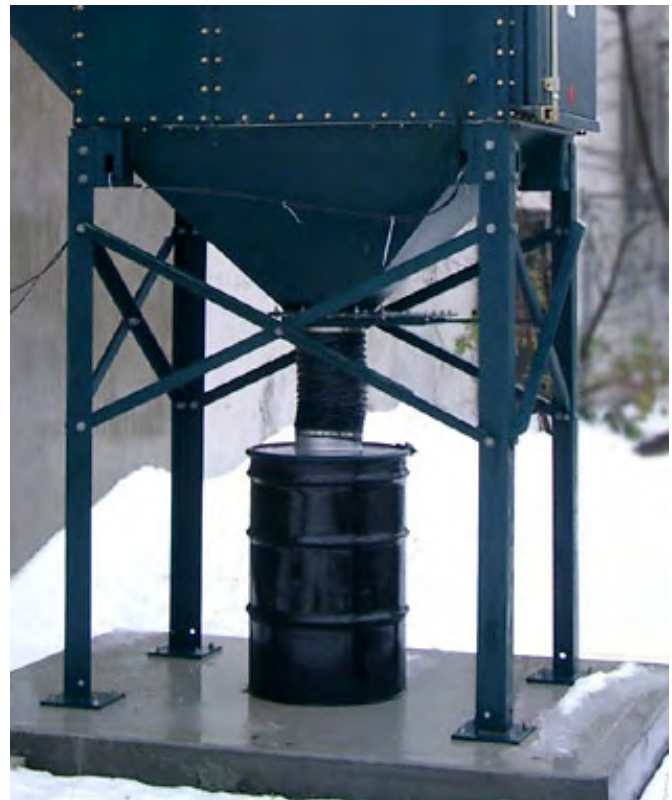
Storage drum prevents dust from backing up in the hopper and creating an explosion hazard.
