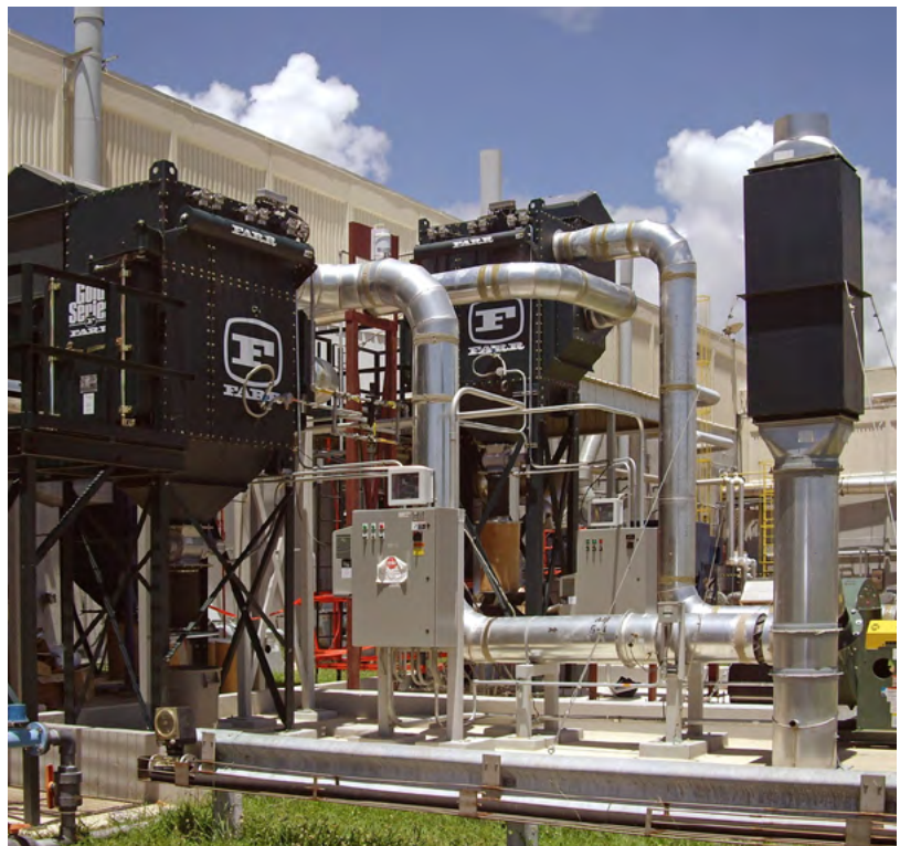
These dust collectors are equipped with passive and active controls. Passive controls are an explosion vent and ducting that control the pressure and flame direction, and a rotary valve that contains the flame in the hopper. The active control is a chemical isolation system mounted on the inlet duct. Triggered by a pressure/flame detector, it will extinguish a flame front passing through the inlet pipe before it goes back into the plant.
